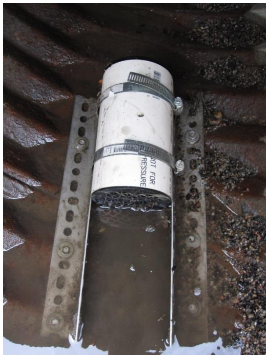
Figure 4-17 Filter Trench Influent Sampler Deployment Unit
